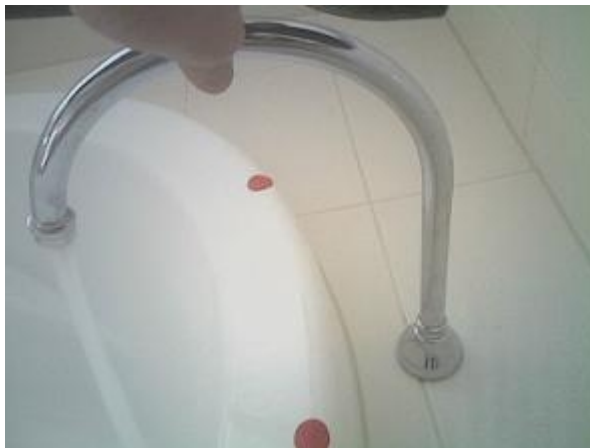
Bath taps Water hammer Major Defect Type: F Water pipe to the bath tub exhibits water hammer. Extensive rectification work will include demolition of wall cladding, re-bracketing of pipes so they are firmly attached to the wall and re-instatement of cladding and finishes including water proofing. Occurs to ensuite.
