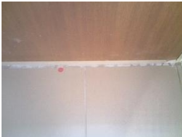
Walls Not straightened prior to plasterboard installation Minor Defect Type: F Wall should have been straightened prior to plasterboard installation.
