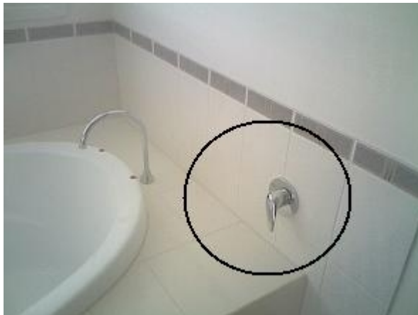
Shower screen Inadequate screen Minor Defect Type: F Shower screen should be replaced as it does not suit the height of the hob. This may be the case on every particular home of this style unless the hob was built to high. Silicone sealant to this height is not acceptable.
