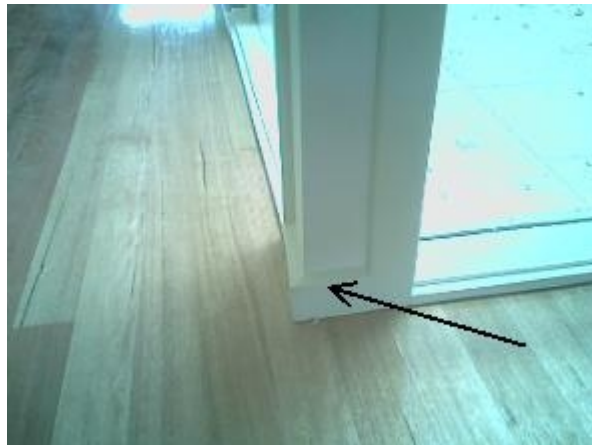
Doors and frames Architraves set at different levels Minor Defect Type: F Architraves to bathroom, Bed 2 & Bed 3 are set at different levels and should be fixed.
