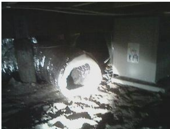
Air conditioning system Ducts run along ground Ducts will decay if left on natural ground.
